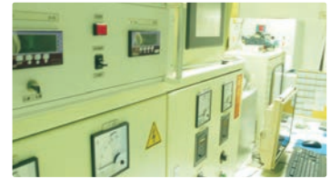
風洞實驗室 LAB OF TESTING FANS
